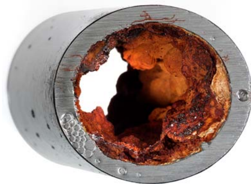
ABOVE: Galvanized steel pipe shows build of mineral and other deposits.
