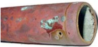
BELOW: Exterior view of pinhole leaks in a copper pipe.
